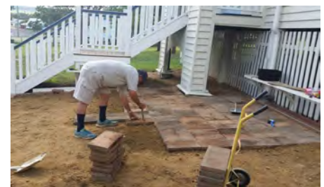
Carlos, hard at work laying pavers to create an attractive outdoor area at the front of the Catholic Church. Perfect spot for a cuppa after church!
